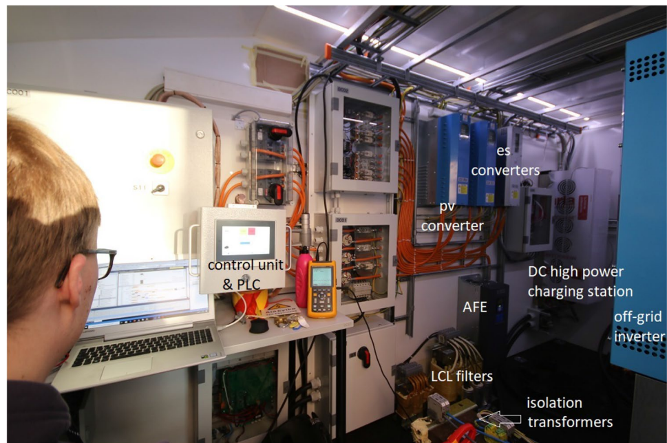
Fig. 3 Overview to power electronics trailer shows how the main components of Fig. 2 have been installed in the trailer. LCL filters are used to remove harmonics
